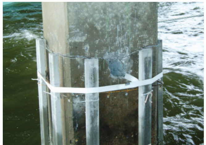
Galvanic anode system on bridge column prior to encasement in concrete jacket.
