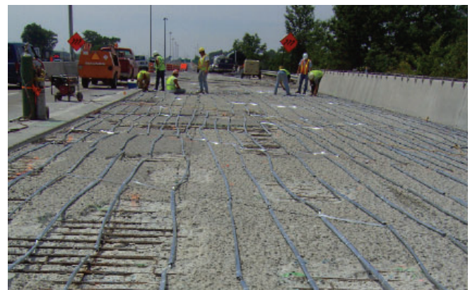
Galvanode DAS Type F distributed anode system on bridge deck prior to placement of reinforced concrete overlay
