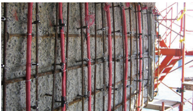
Galvanode® DAS Type C distributed anode system on corroded abutment prior to encasement with new concrete.
